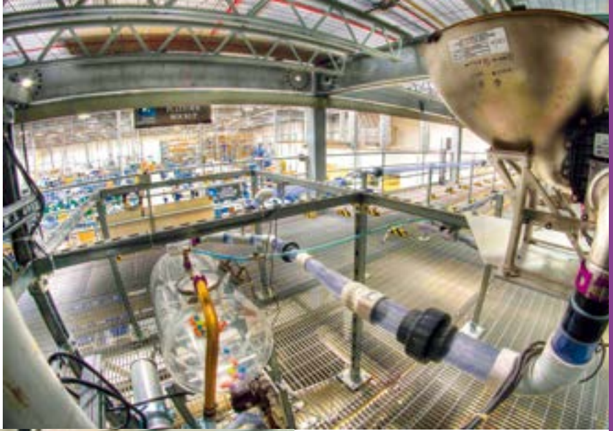
Integration bench for aircraft water and waste systems at the Zodiac Water & Waste Systems division (Carson, California).
